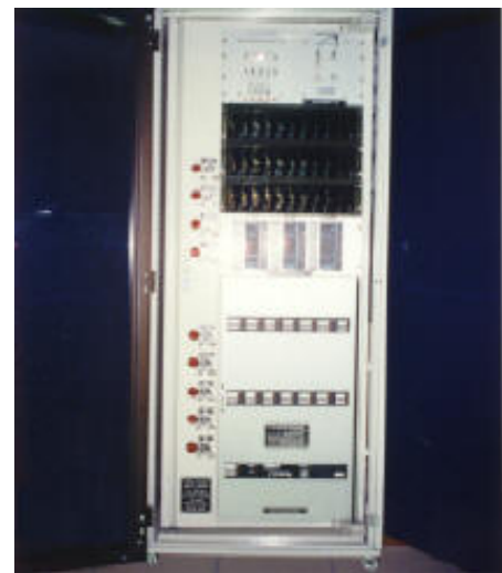
Custom Fire/Gas Safety Panel
